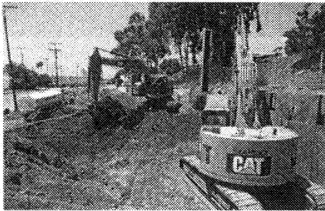
Excavation in preparation for construction of the piles and footings for the bridge abutment expansion
